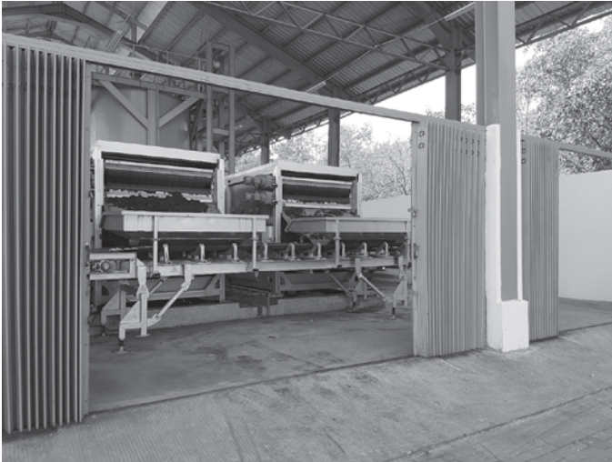
Photo 7.4 Belt filter press at Duri Suwung Septage Treatment Plant, Denpasar, Indonesia Source: Chengyan Zhang of Stantec
