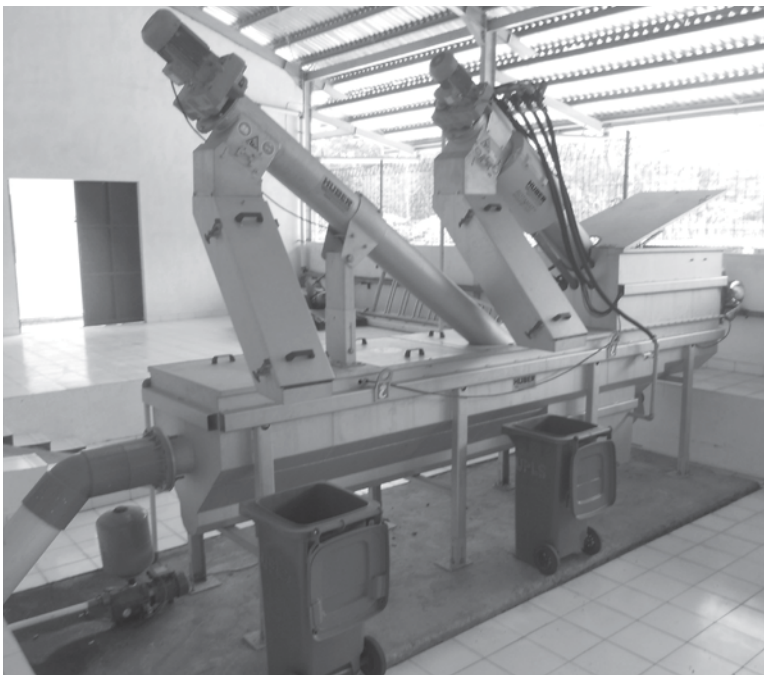
Photo 6.8 Combined mechanical screening and grit removal, Jakarta
