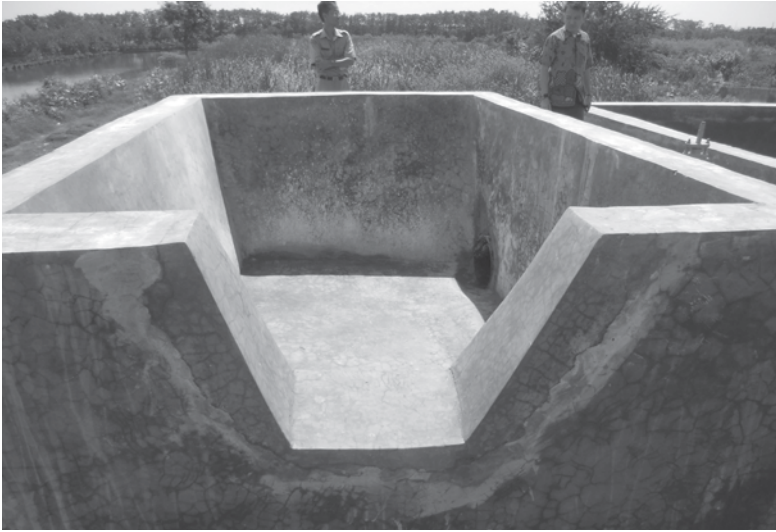
Photo 6.2 Septage reception chamber, Tegal, Indonesia
