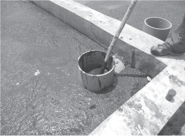
Photo 5.4 Blocked connection pipework
