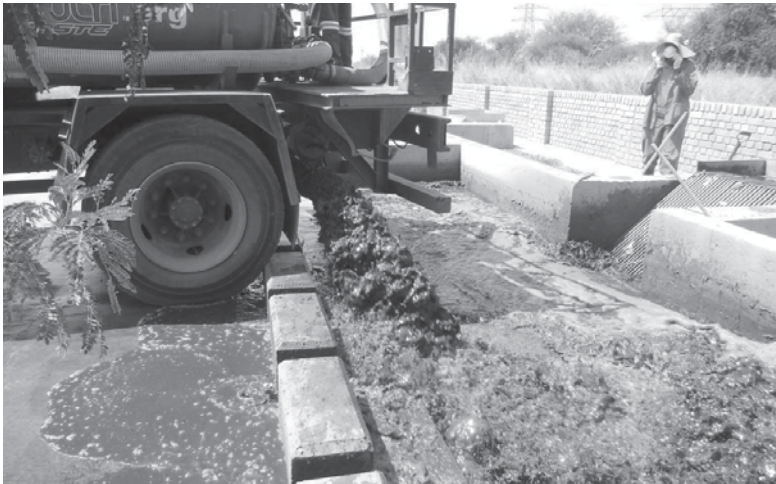
Photo 6.3 Flat apron receiving unit that could be improved by adjusting the levels so that the apron is lower than the road, Gaborone, Botswana
