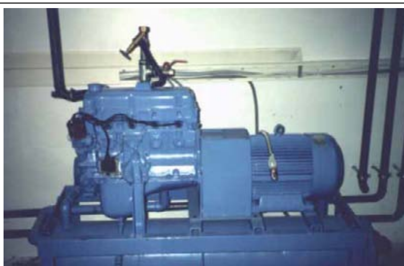
Figure 47: Co-generation unit (electricity and heat utilisation)
