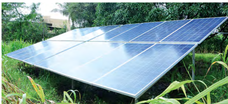
Figure 5.9 Array of solar PV modules (Promethean).
