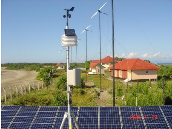
Wind, 5kWp -Solar, 5kWp Hybrid System at St. Martins Island, Cox's Bazar, Bay of Bengal, Bangladesh
