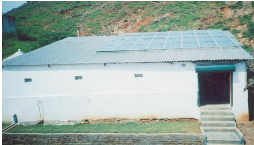
SOLDRY- FISH PROCESSING FACILITY PLANT, AT DFYWA, VISAKHAPATNAM
