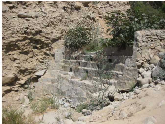
Figure 7: An example of a Peruvian stone wall constructed in the last decade to dissipate energy from landslides moving down the Rimac River. Intake structures can be constructed in a similar way. Photo: Sakthy Selvakurmaran.
