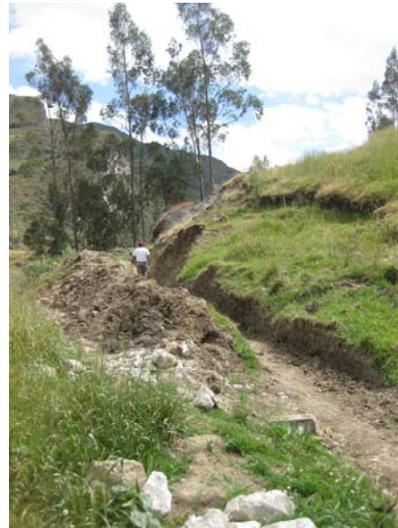
Figure 4: The diversion channel at Yanacancha after a slope collapse – faults due to soil creep are clearly visible. Photo: Sakthy Selvakurmaran.
