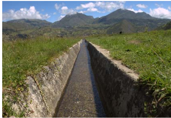
Figure 2: One of the concrete lined channels. These are built very cheaply with no shuttering, minimal expansion joints and thickness of just 50 – 75 mm. Photo: Sakthy Selvakurmaran.
