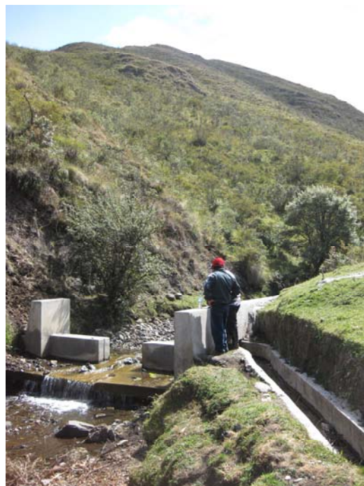
Figure 1: The intake structure with stoplogs removed at El Regalado. The structure is made with reinforced concrete and erosion on the channel side slopes is visible. Photo: Sakthy Selvakurmaran.
