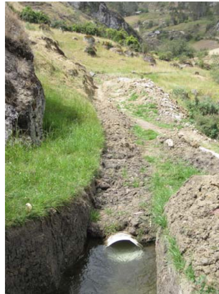
Figure 5: Buried pipe can be used to replace channels that have been destroyed by slope collapse but this is expensive. Photo: Sakthy Selvakurmaran.
