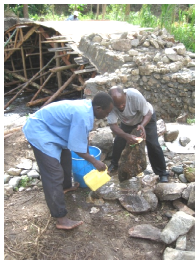
Fig. 45: The use of a gauged batch box and ruler is a precondition for producing quality mortar. Basins and wheel barrows should not be used as it is difficult to control the exact amounts.
