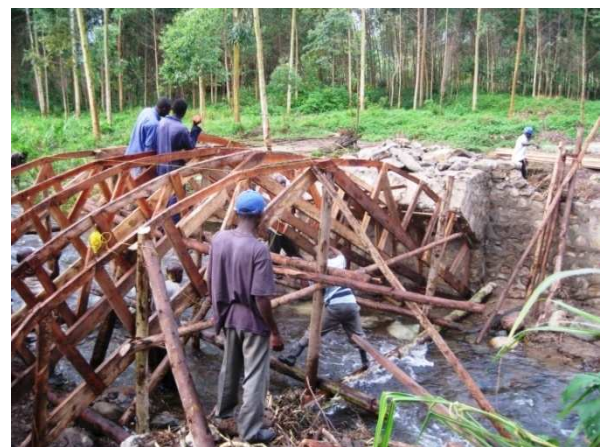
Fig 29: five trusses are required for a standard width of 3.6 m. The trusses are supported by struts.
