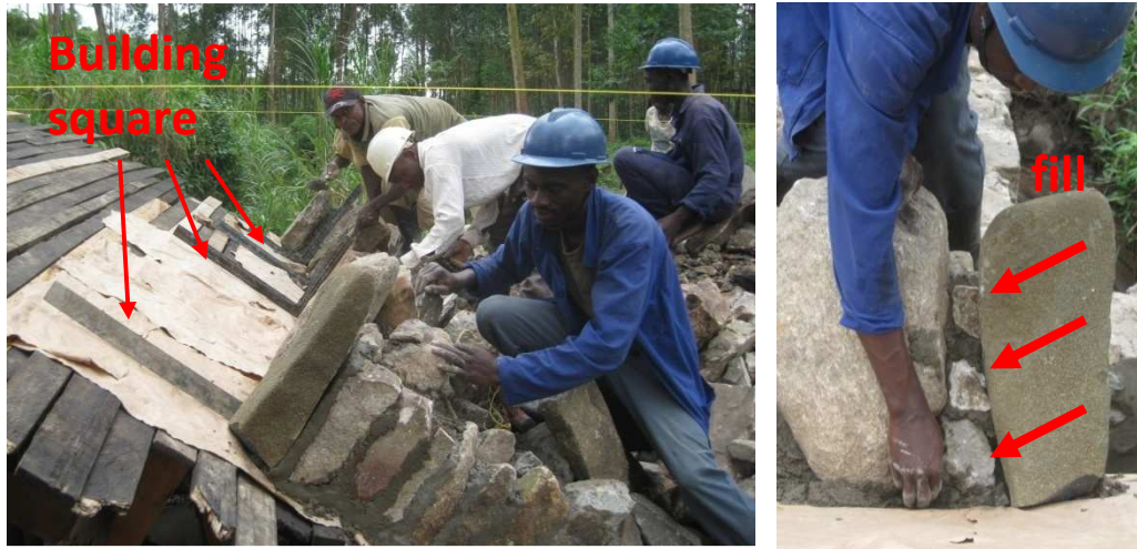
Fig 38: Left: Building squares show the right position of the stones during each phase of the arch construction. Right: It is of utmost importance to fill all gaps between the stones. Small stones will be added to the mortar to reduce cement costs and increase strength.
