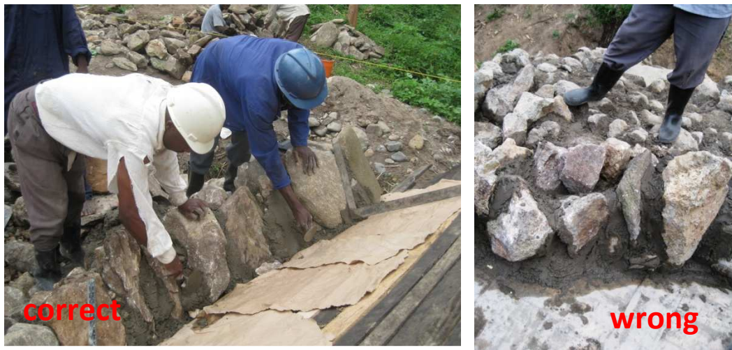
Fig 39. The quality of the craftsmanship is of extreme importance for the strength of the arch. Left: Good bond and proper positioning of stones. Right: poor stone masonry that will result in a weak structure.
