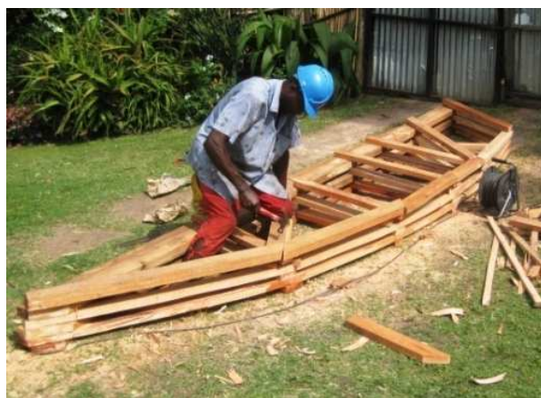
Fig. 28: Once the first mould is constructed, the others are easily copied and shaped with a machete.
