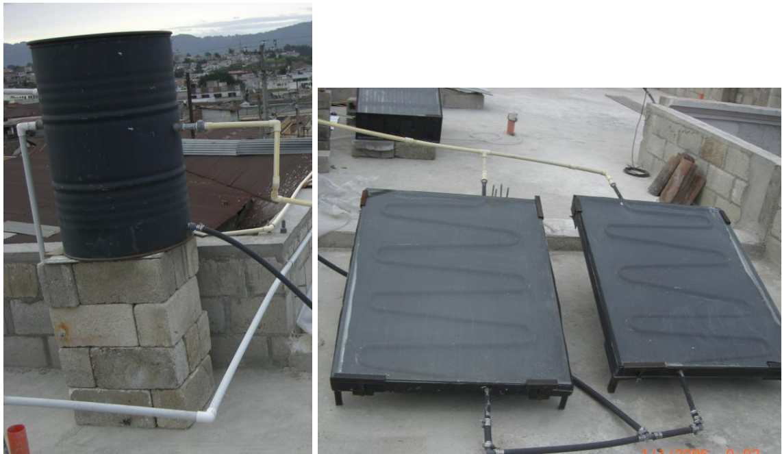
Solar Serpentine System at AIDG Guatemala
