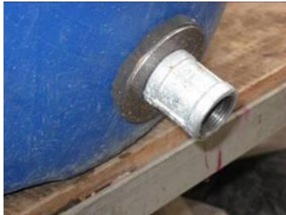
Inner hot water tank: bulkhead fitting (outside the tank)
