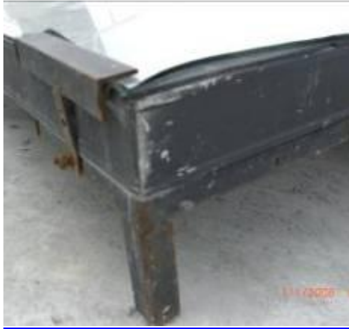
Bottom of Collector Brackets
