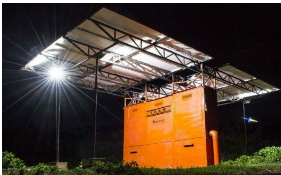
Figure 9: Solar PV power station using SteamaCo technology. Credit: SteamaCo
