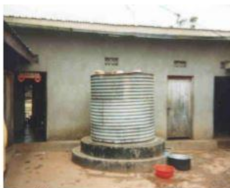
Figure 4b: A corrugated iron RWH tank in Uganda
