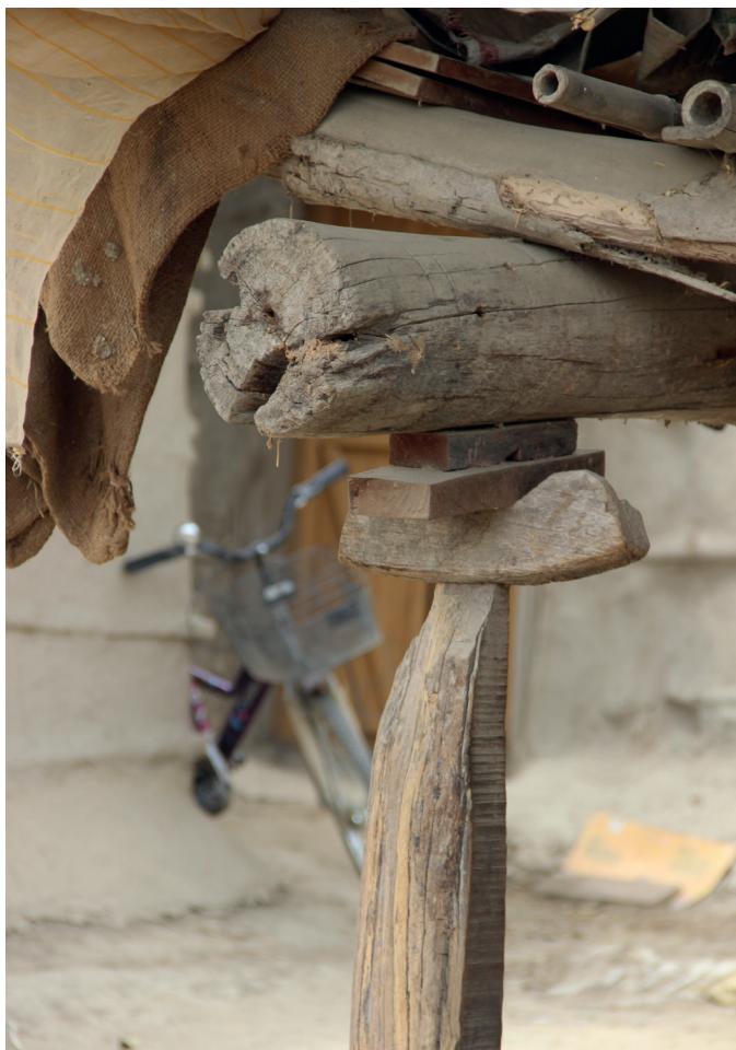
Figure 8: Ad-hoc timber construction. This image demonstrates a number of important points, the lack of availability or access to appropriate timber in long enough lengths, the use of random pieces of timber to provide additional height and little or no skill in carpentry to make an effective joint.
