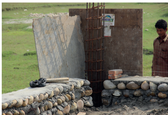
Figure 11: Building under construction. Note the ad-hoc, poorly constructed formwork and inadequate reinforcement. The local supply of materials was limited to smaller diameter, plain (non-deformed) bars with little attention to the use of steel links. Scrap timber boards are used to contain wet concrete, with little or no effective carpentry in evidence.
