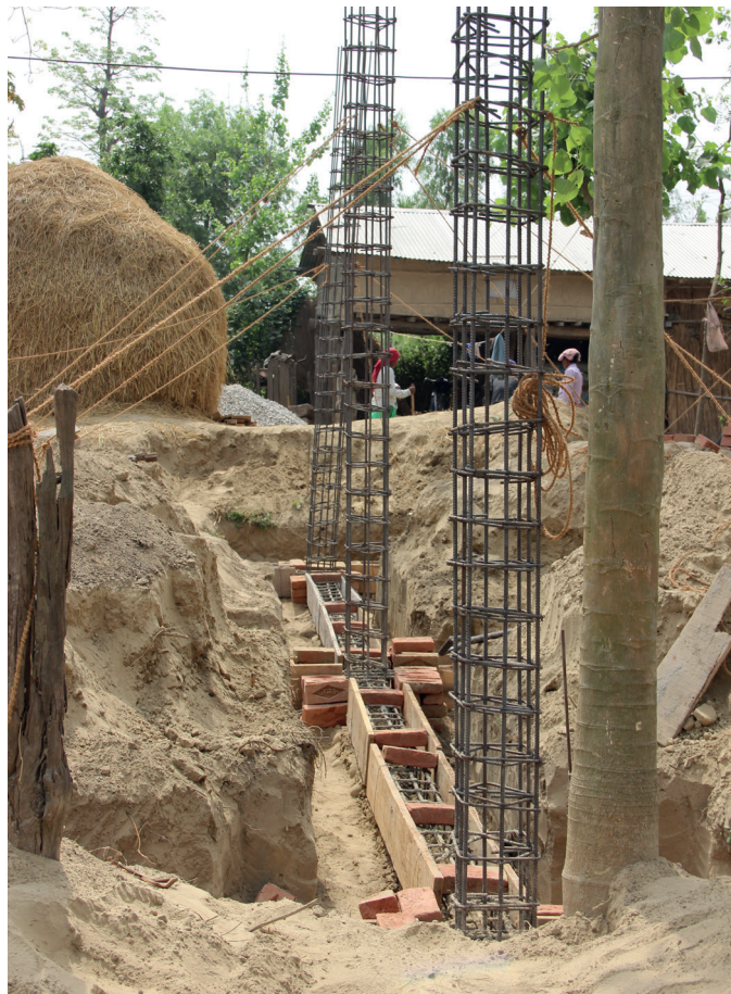
Figure 9: Engineered reinforcement for flood refuge shelters. Eight deformed steel bars, which have a rippled surface to attach more effectively to the concrete, are tied at frequent intervals with horizontal steel links for a robust structure. This type of reinforcement did not seem to be available at the local suppliers we visited.'
