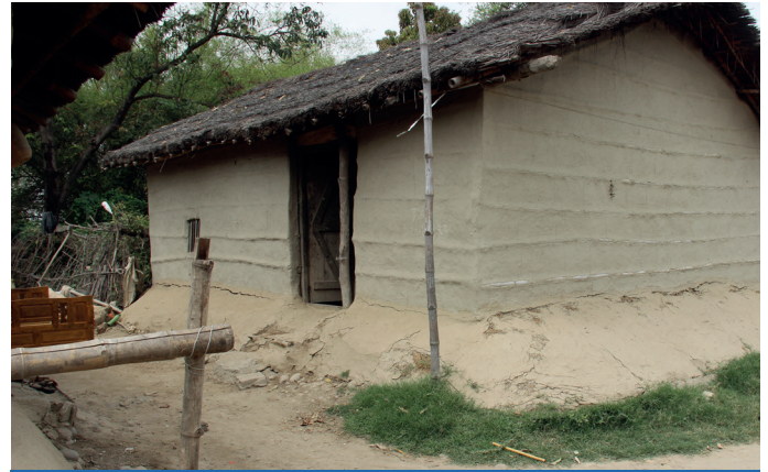
Figure 7: House with limited resilience, located less than 50 metres from the river. Constructed of timber, bamboo and earth, it sits on a slightly raised platform below the levels reached by water during flooding.
