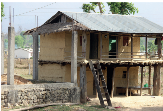
Figure 10: A new concrete house being built adjacent to a traditionally flood resilient house. Note the raised plinth platform and concrete pillars. Concrete represents a considerable financial investment compared to vernacular construction and may be perceived by local communities to be more resilient.
