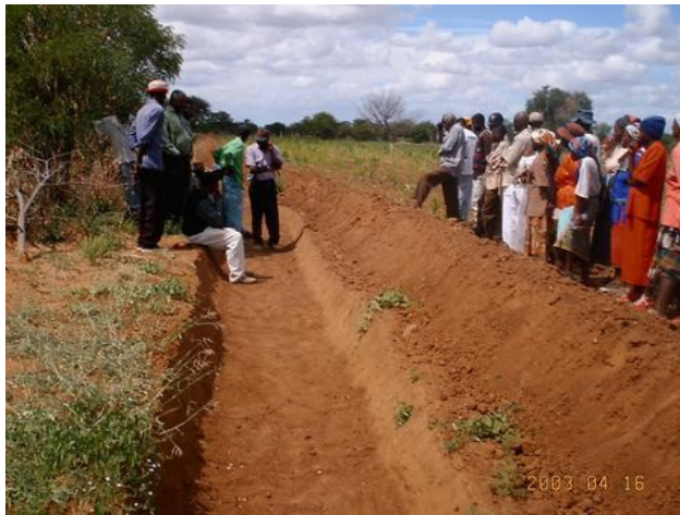
Figure 2: Complete dead level contour ready to harvest water. Photo: Practical Action, Southern Africa.
