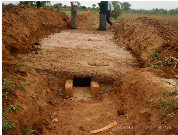
Figure 3: 10 m 3 water storage facilities to avoid evaporation & deep percolation Photo: Practical Action, Southern Africa.
