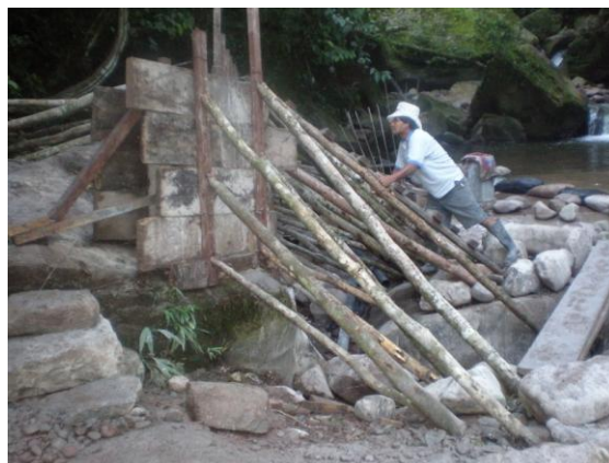
Figure 3: Civil engineering for a micro hydro scheme in Bocatoma, Peru. Photo: Soluciones Prácticas.
