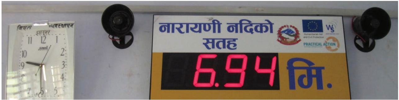
Photo 9: Electronic display of flood level at CDO Office, Narayani
