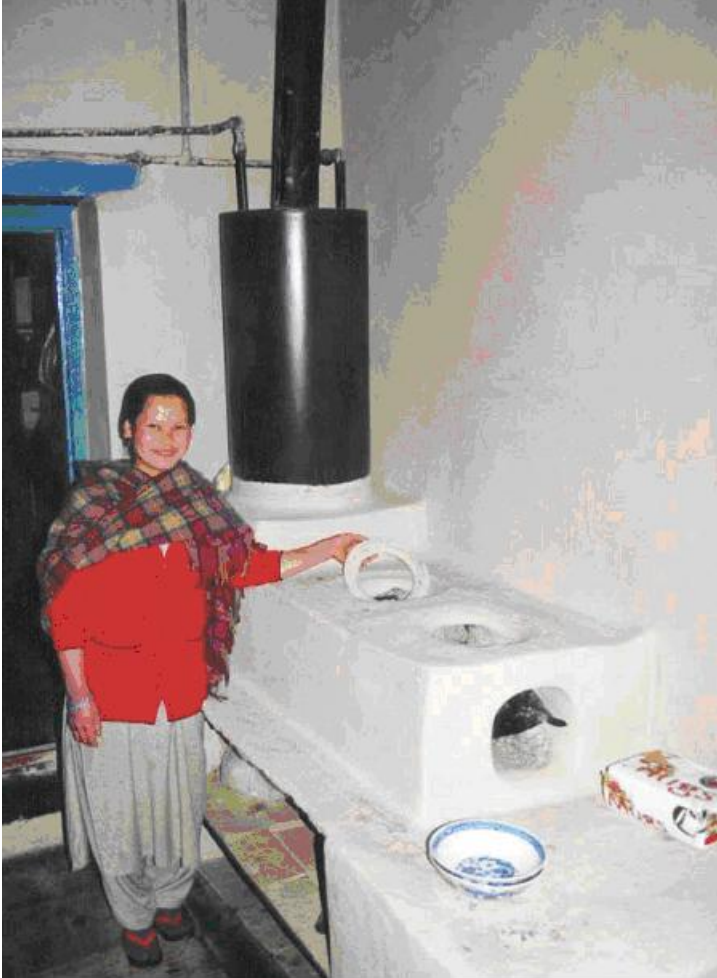
Smoke water heater in a hotel restaurant in Jomsom.
