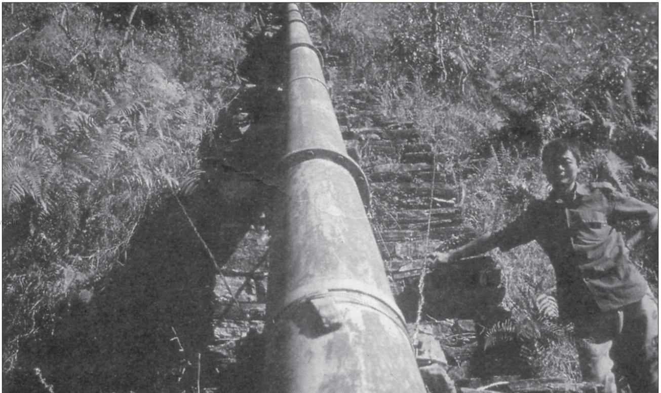
Photo 9.4 Stone masonry can provide slope stabilisation along the route of the penstock (Barpak)
