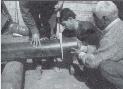
Photo 4.21 Joining HDPE pipes by pushing them while hot. Notice the Teflon bag.
