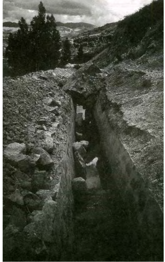
Photo 2.2 Obstruction caused by debris falling from on unstable slope
