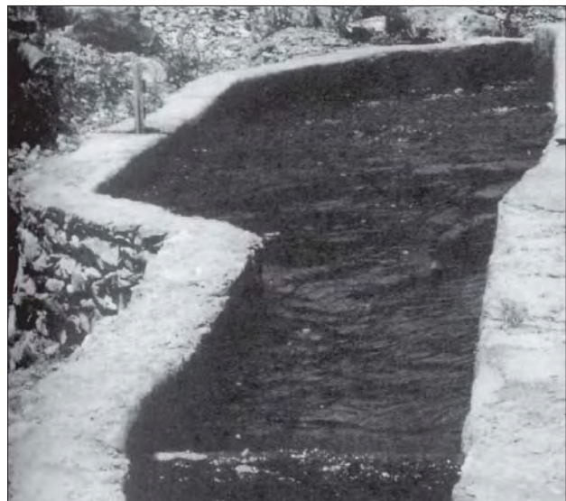
Photo 5.1 Galkot gravel trap
