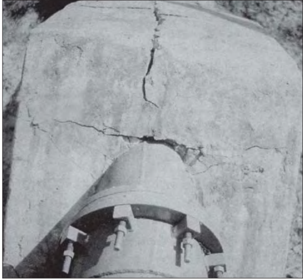
Photo 7.3 Cracking of the upper surface of an unreinforced anchor block
