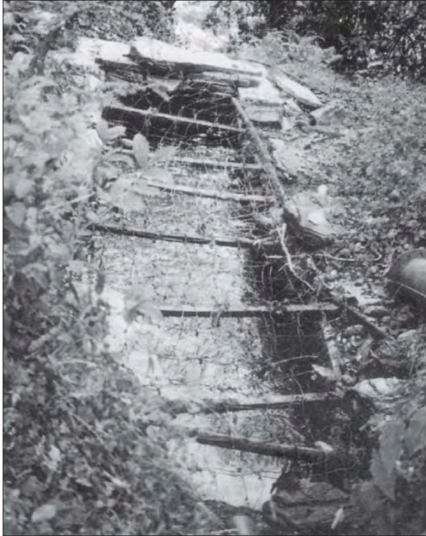
Photo 5.7 Ghandruk settling basin
