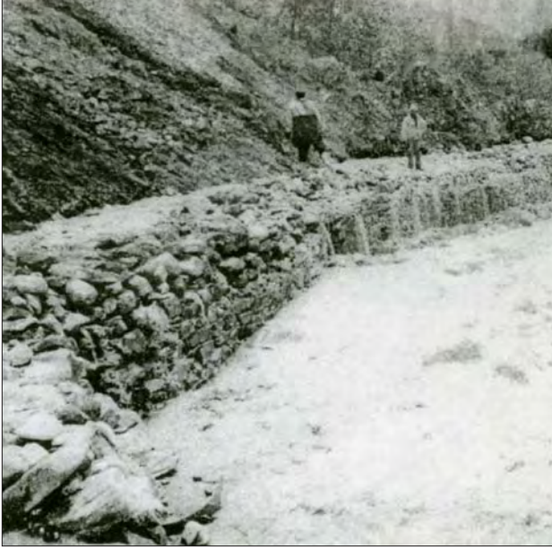
Photo 3.11 Gabion walls at the headworks of the 30kw Jharkot micro-hydro scheme, Mustang, Nepal.
