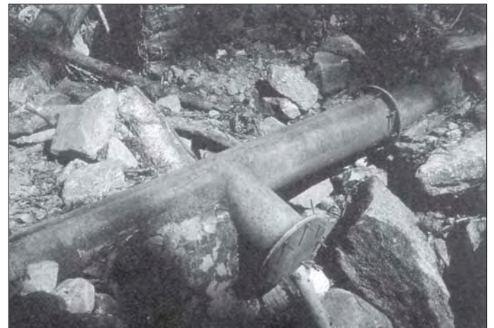
Photo 4.17 Flush-outs should be provided at low points in pipelines so that heavy debris can be periodically removed (Siklis)
