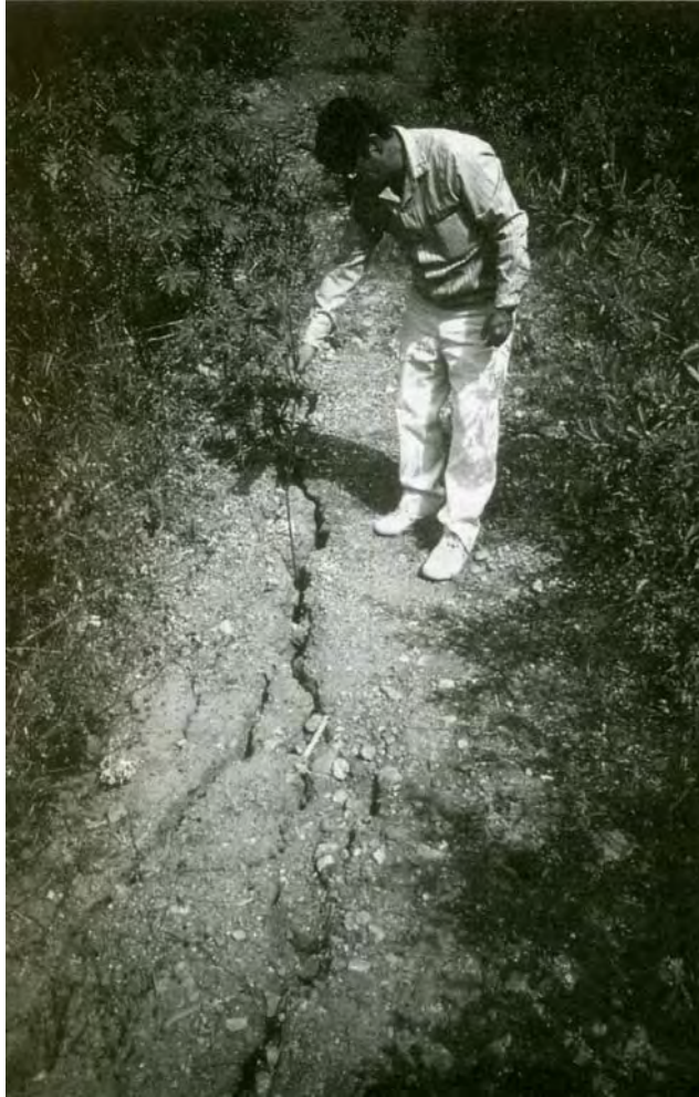
Photo 2.1 Tension cracks along a slope
