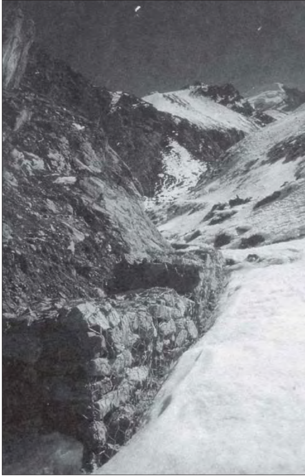
Photo 9.3 Gabion at the toe of an unstable slope
