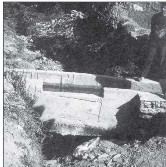
Photo 4.12 Spillway on a crossing where the excess flow is discharged into a gully, Galkot micro-hydro scheme, Baglung, Nepal.
