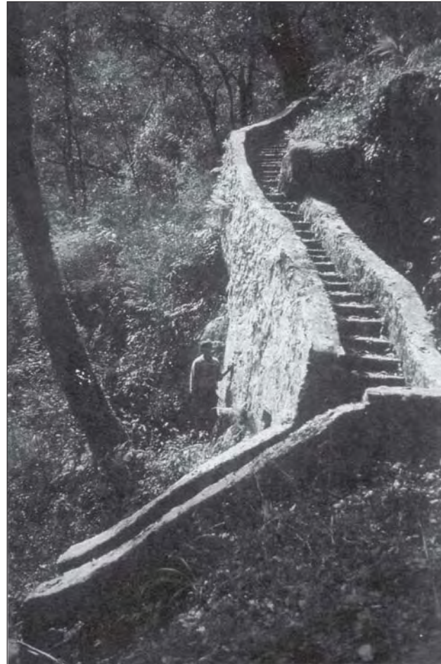
Photo 9.2 Masonry steps for energy dissipation and control of spillway water. Although costly, elaborate control is essential where slopes are vulnerable to erosion (Sikkis)
