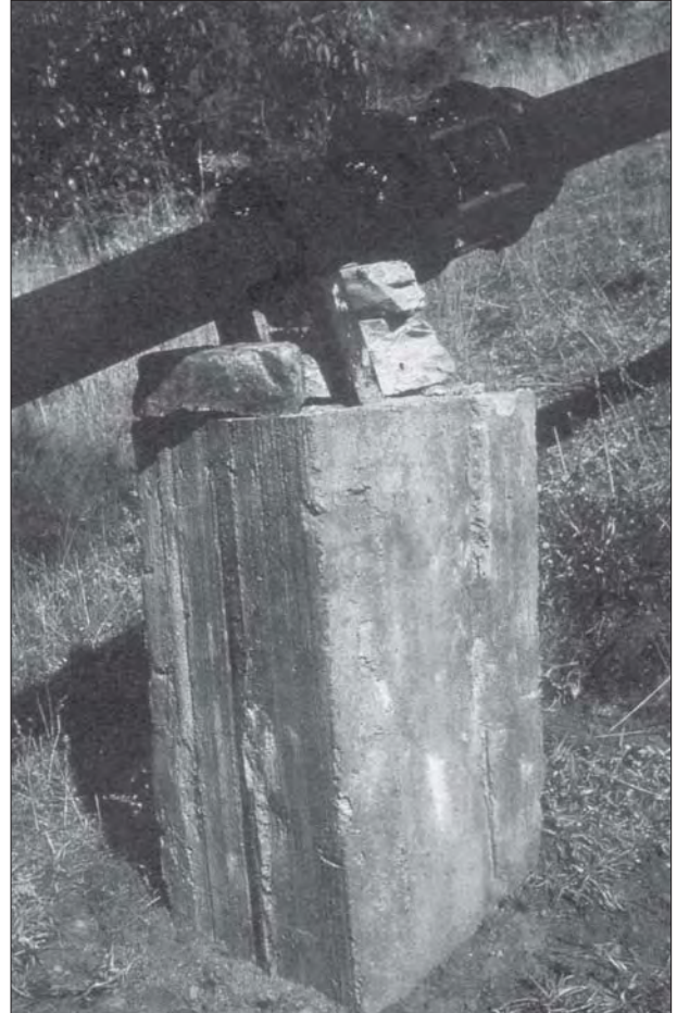
Photo 7.6 The use of an extension to the concrete support lifts the pipe clear of a block, allowing drainage and preventing corrosion between the block and the pipe (Khamche)
