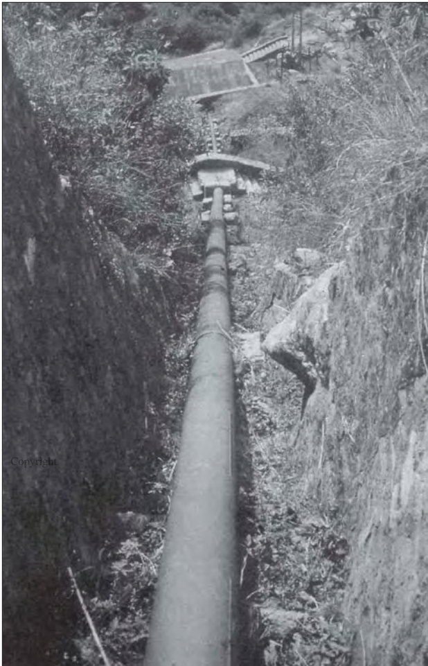
Photo 6.3 Excavation to reduce the cost of the penstock and reduce the need for anchors (Siklis)
