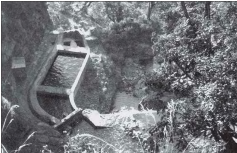
Photo 5.8 Gravel trap, settling basin and forebay of Jhankre mini-hydro
