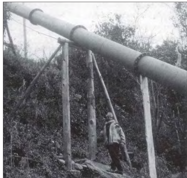
Photo 7.7 Wooden support piers at Kamche micro-hydro, Nepal
