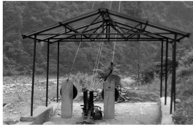
Photo 6: A down hill ropeway station in Fisling, District Chitwan
