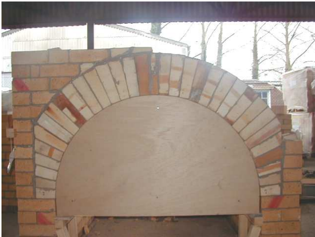
Figure 3.6: Primary chamber access arch construction (with former in place) from the Ash End
