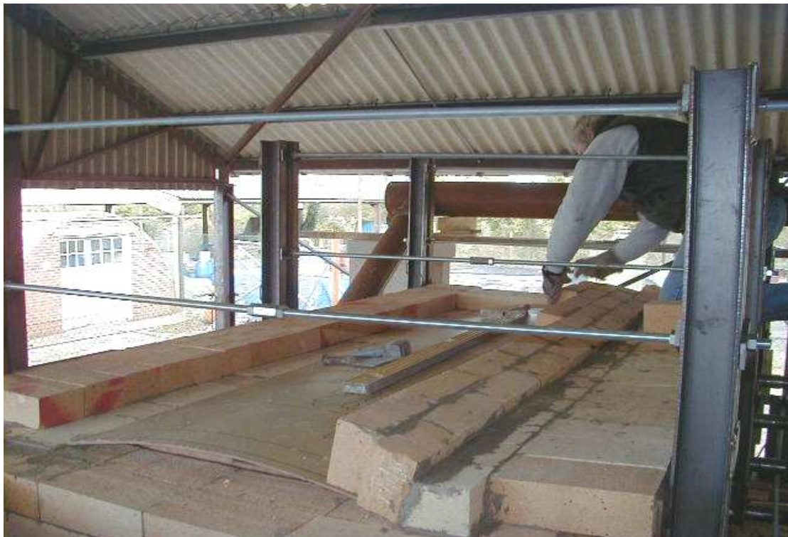
Figure 3.16: Secondary chamber roof-arch under construction – showing arch former and backstays in position
