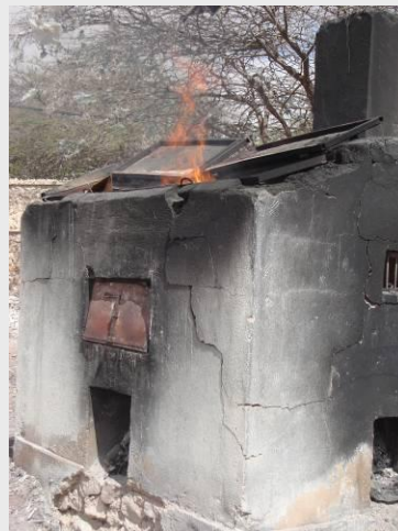
Fig. B.1 – Old incinerator used at General Group Hospital before the intervention
