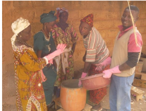
Figure 7: Women are learning how to apply the cement layer during a workshop. Photo credit: Movement e.V. / Peter Rinker.
