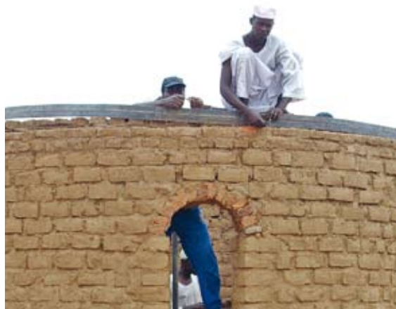
Pic 11. Two courses of red bricks are laid on top of the green bricks
