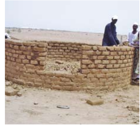
Pic 7. The wall is built up leaving a gap for the door
