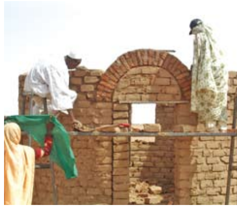
Pic 9. The door arch using method 2; a girder made from bricks and muna
