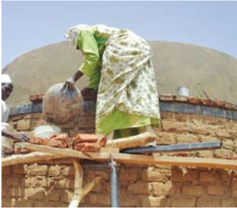
Pic 18. A course of red bricks act as a gutter
