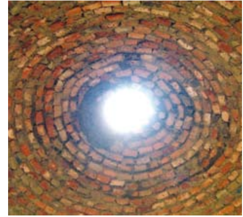
Pic 20. The dome roof from inside, a small hole is left in the top for ventilation
