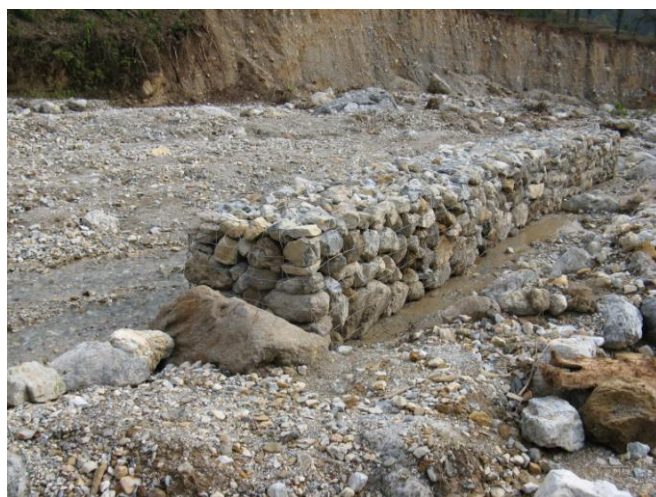
Figure 6: An example of a spur that has not been installed with groundwork or an apron and consequently is likely to be washed away during heavy flooding. Photo: Practical Action Nepal.
