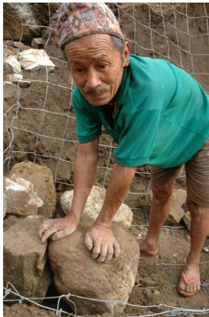
Figure 12: Loading rocks into the gabion cages, a community activity. Photo: Practical Action Nepal.
