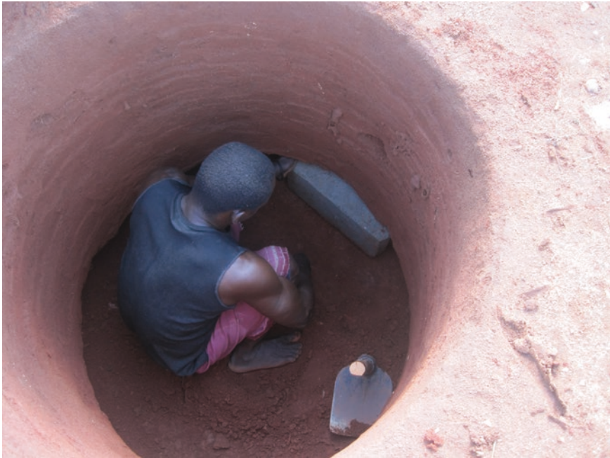
Photo 6.1 Small diameter well-digging and underlining for additional shaft support Source: Photo H. Holtslag
