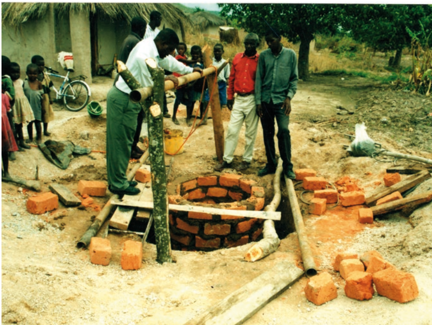
Photo CS.6.1 Family well upgraded in Northern Province Zambia using the training from Mvuramanzi Trust, Zimbabwe
