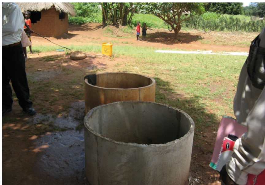
Photo 6.6 Concrete well rings for traditional family well improvement (well in background) Luapula Province, Zambia
