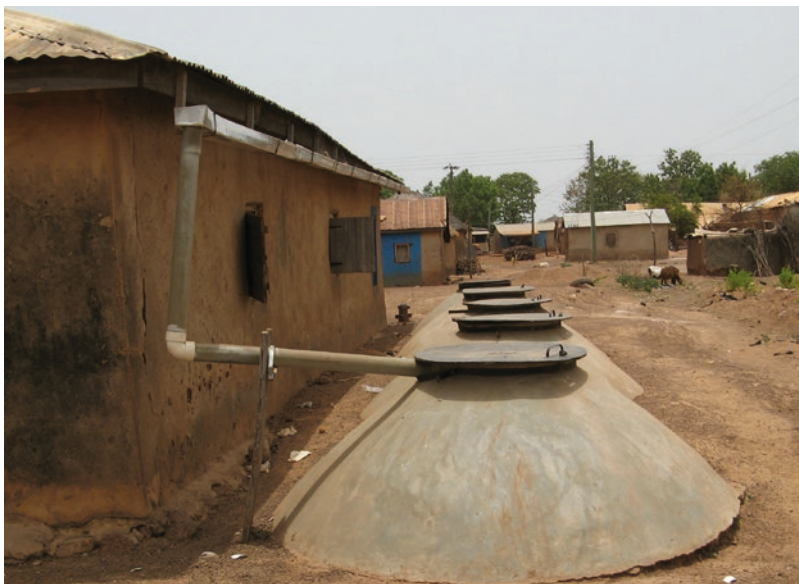
Photo 6.18 High cost expansion of rainwater in-series storage, Ghana
