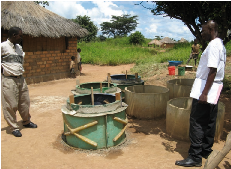
Photo 9.1 Well-lining rings made by local artisans at Sila Mumba's house (Existing well head in the background)
