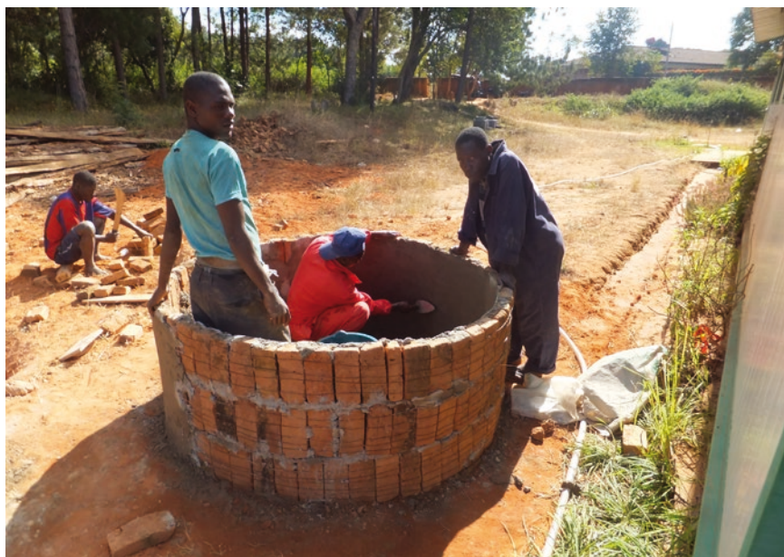
Photo 6.19 Constructing domestic wired-brick rainwater storage with cement lining, Malawi Source: Photo R. Veldman, SMART Centre Group
