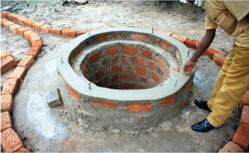
Photo 6.5 Brick lining for well and drainage channel (part completed) with foundation for top slab, Northern Province, Zambia
