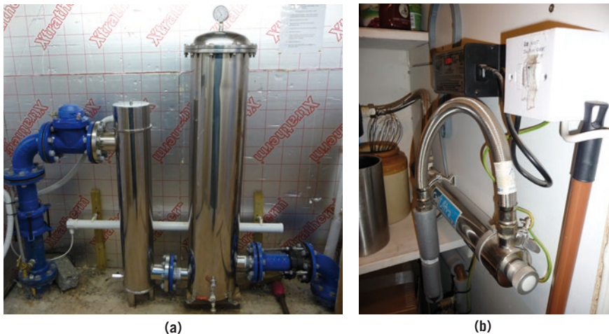
Photo CS.1.2 Two private water supply treatment systems: (a) supplying a large estate and (b) a simple 'point of use' ultraviolet disinfection unit in a kitchen cupboard Source: DWQR
