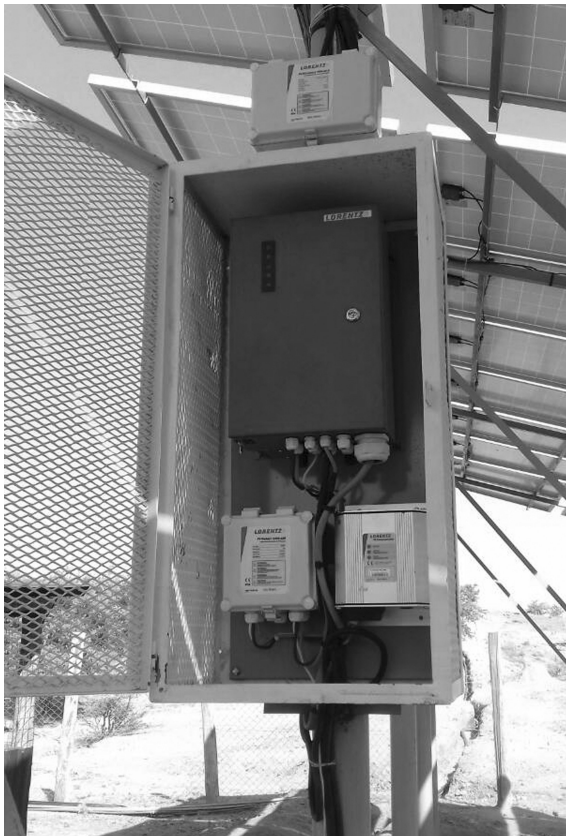
Figure 6.5 Inverter installed in a lockable meshed enclosure under the PV array at Turkana, Kenya Source: Oxfam
