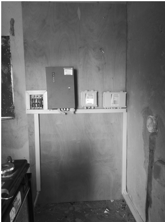
Figure 6.4 Installed controls (left to right): AC changeover switch, inverter, surge protector, PV disconnection switch
