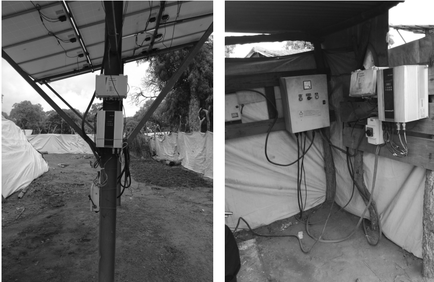
Figure 6.6 Examples of poor cable management in South Sudan
