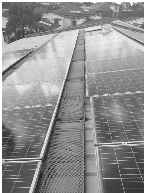
Figure 6.18 Walkway on a roof mount at Strathmore University, Kenya
