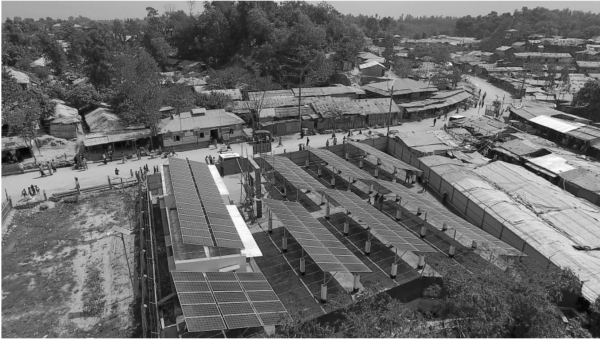
Figure 6.11 Combined roof and pole mount installation at IOM water scheme, Kutupalong Balukhali Expansion Site refugee camp (Cover photo) Source: IOM-Bangladesh
