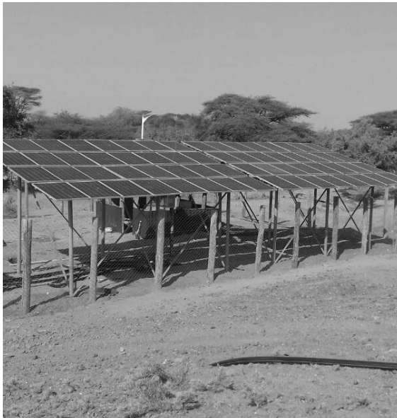
Figure 7.3 Fenced SPWS with a solar light for security in Turkana, Kenya
