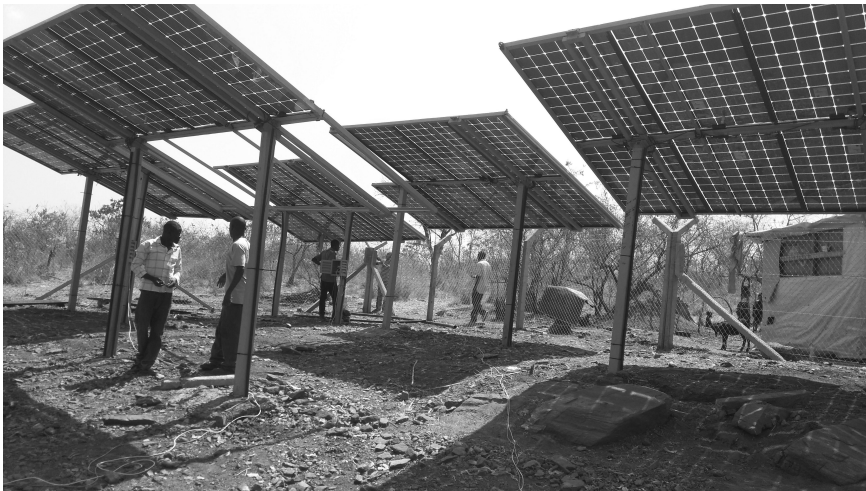
Figure 6.9 Pole mounted PV modules in Bidibidi refugee settlement, Uganda
