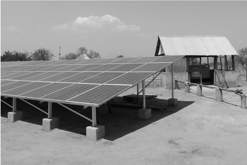
Figure 5.9 Hybrid solar-generator scheme at Adjumani refugee settlement in Uganda Source: Oxfam, 2016
