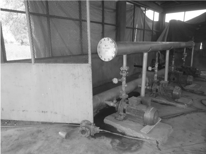
Figure 6.3 Horizontal surface pumps installed on a concrete plinth in Itang Water Supply, Ethiopia
