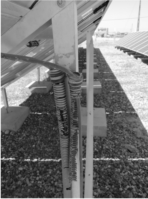
Figure 3.9 Worn-out conduit due to high temperatures in Iraq
