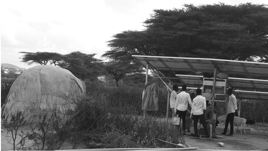
Figure 5.8 Inverter box located under modules in Somali Region, Ethiopia
