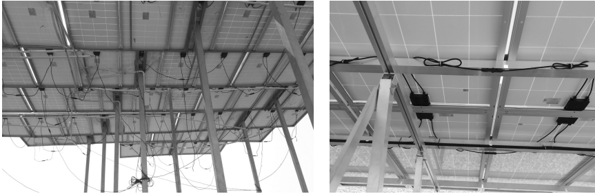
Figure 6.17 Example of untidy and tidy module cables
