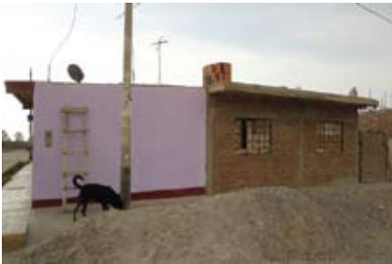
Figure 13.5 Extension of a well-finished improved quincha house with one part made of bricks and a structural frame of concrete
