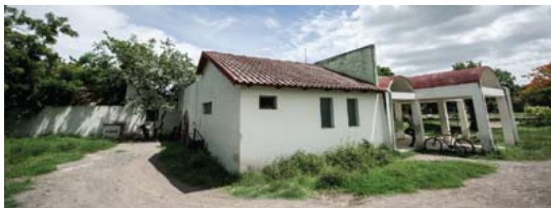
Figure 11.8 Community buildings are well maintained and their tile roofs are in good shape
