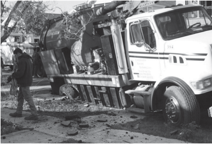
Figure 1 Sinkhole in New Orleans during cleanup
