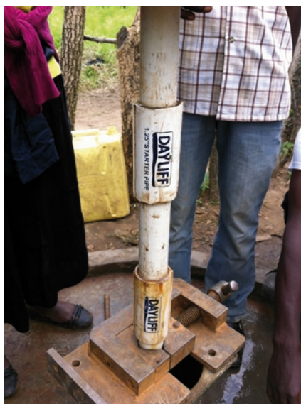
Figure 7 PVC riser pipe fitted to an India MkII pump at Angodingod
