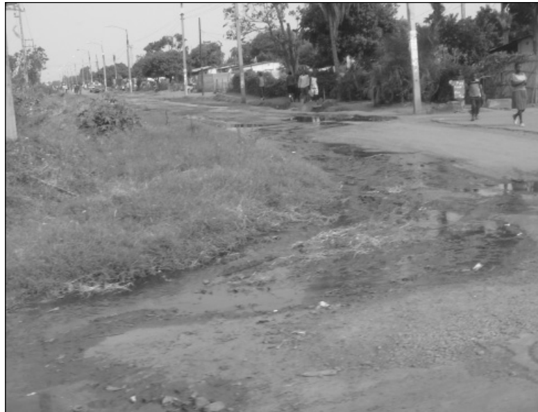
Water from a burst sewer flooded the road
