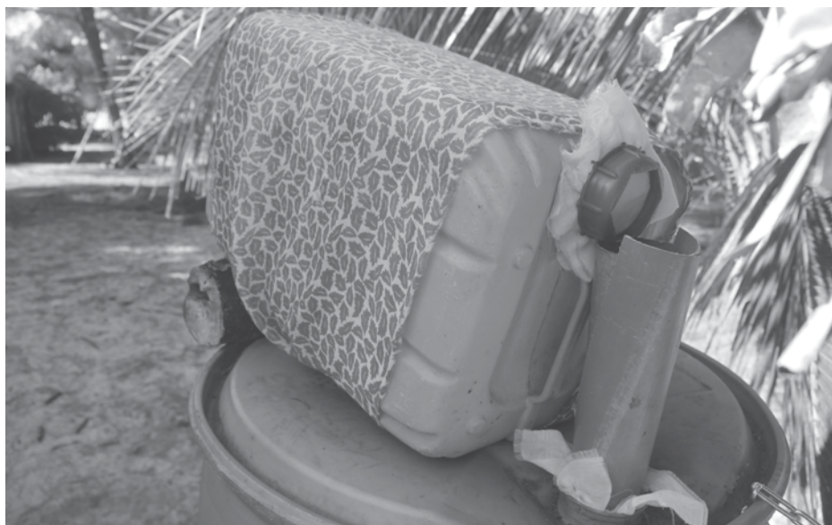
Photo 1 Jerrycan first flush system positioned to convey water to the tank
