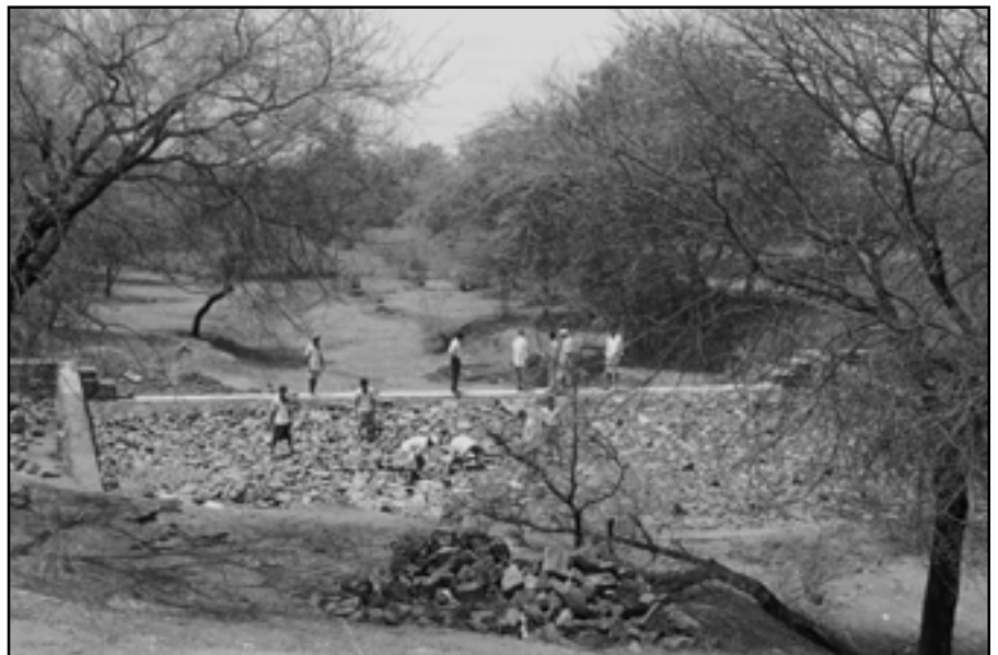
CSE has argued that local water management – such as building check dams like these – can only be done with community participation
